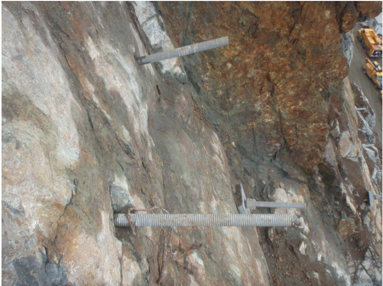
Figure 1. Anchors with no plates or grout on Cut 9, Segment 1. These anchors are to be tensioned rock bolts.
