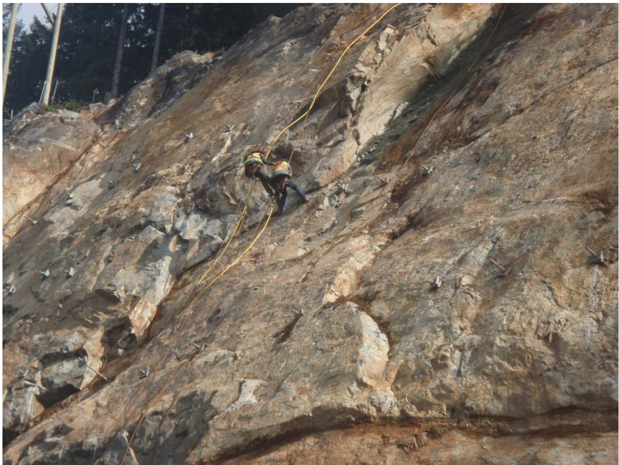
Figure 3. Cut 9/Segment 1. Photo taken one hour prior to the scalers being struck by rock.
